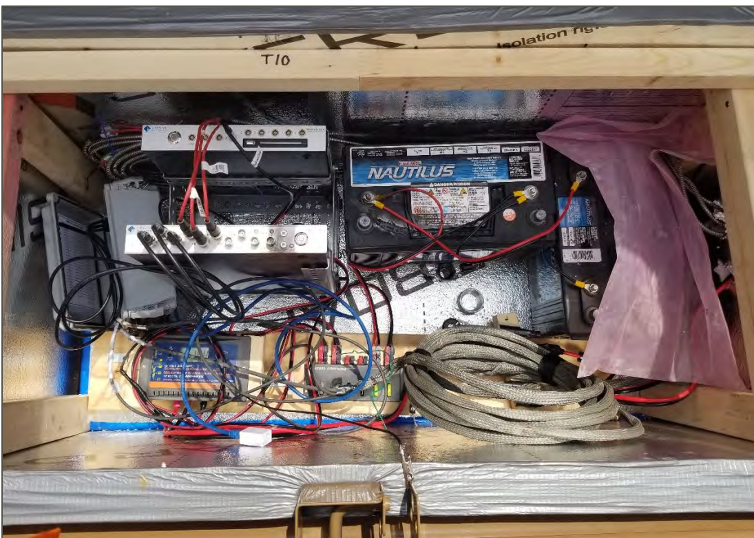
Photograph 8: T10/11 Mock Well data logging and solar power controls inside protective steel box.
