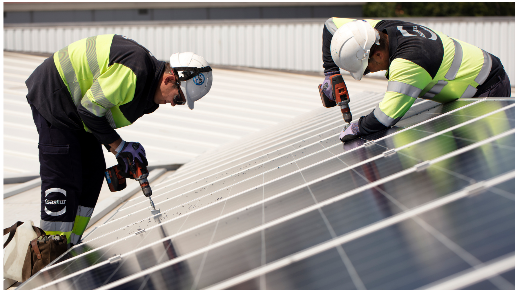
Image: Photovoltaic installation at the Más y Más logistics centre in Spain, supporting the delivery of sustainable energy solutions for business customers.
