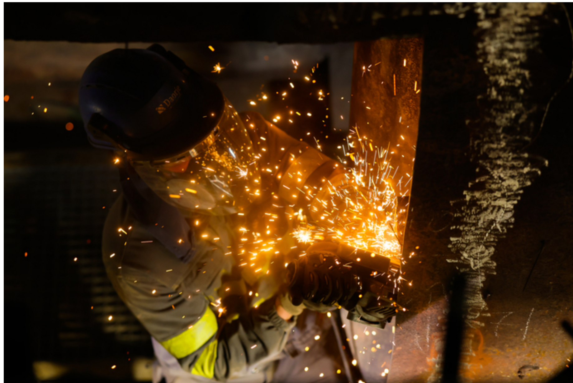
Image: Conversion works at Aboño Power Plant as part of its transition to natural gas generation.
