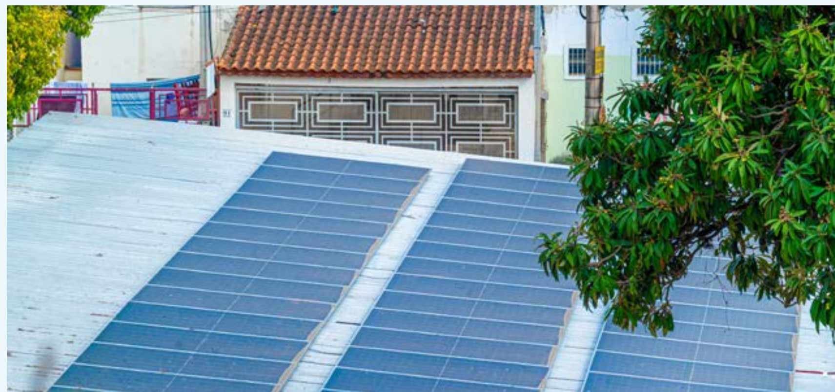
Installation of a photovoltaic solar system at Escola Estadual Ernesto Quissak with 27 kWp of installed capacity.
