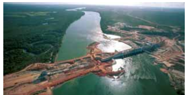
Peixe Angical Hydroelectric Development
